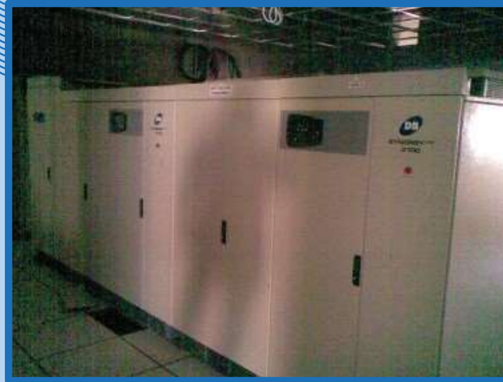
GMR Power Project, Vemagiri, AP
