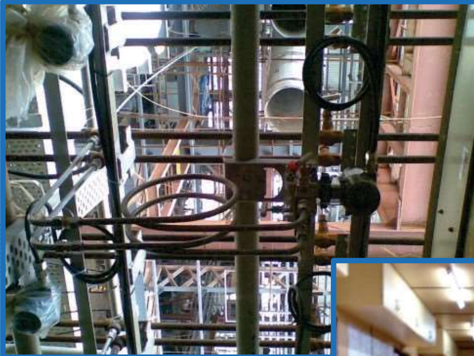
GMR Power Project, Vemagiri AP
