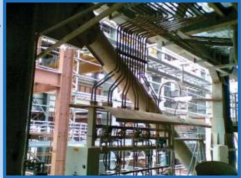
GMR Power Project, Vemagiri, AP
