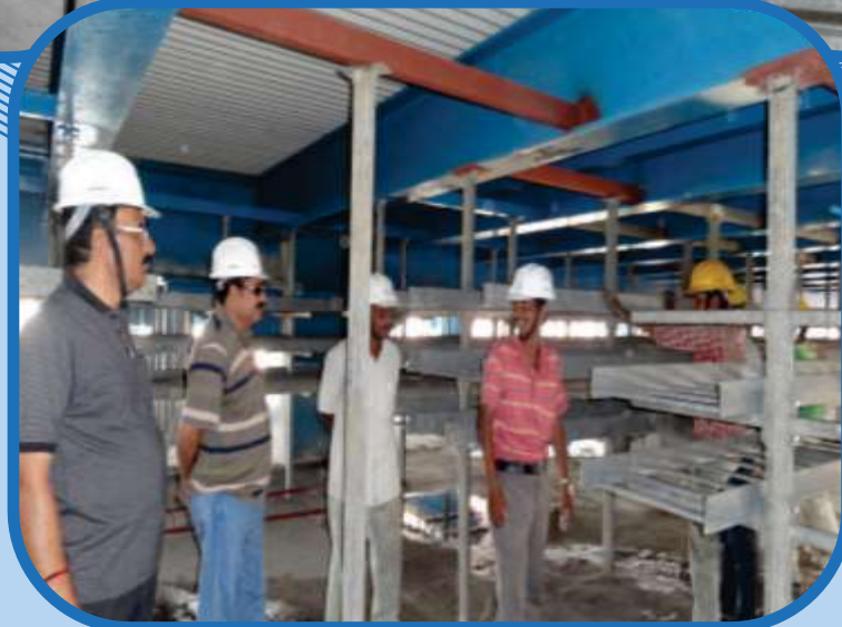
Jimdal Power Plant 600 MW x 4-1 & 2 Unit, CG
