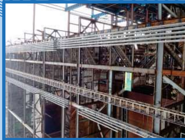
Jimdal Power Plant 600 MW x 4-1 & 2 Unit, CG
