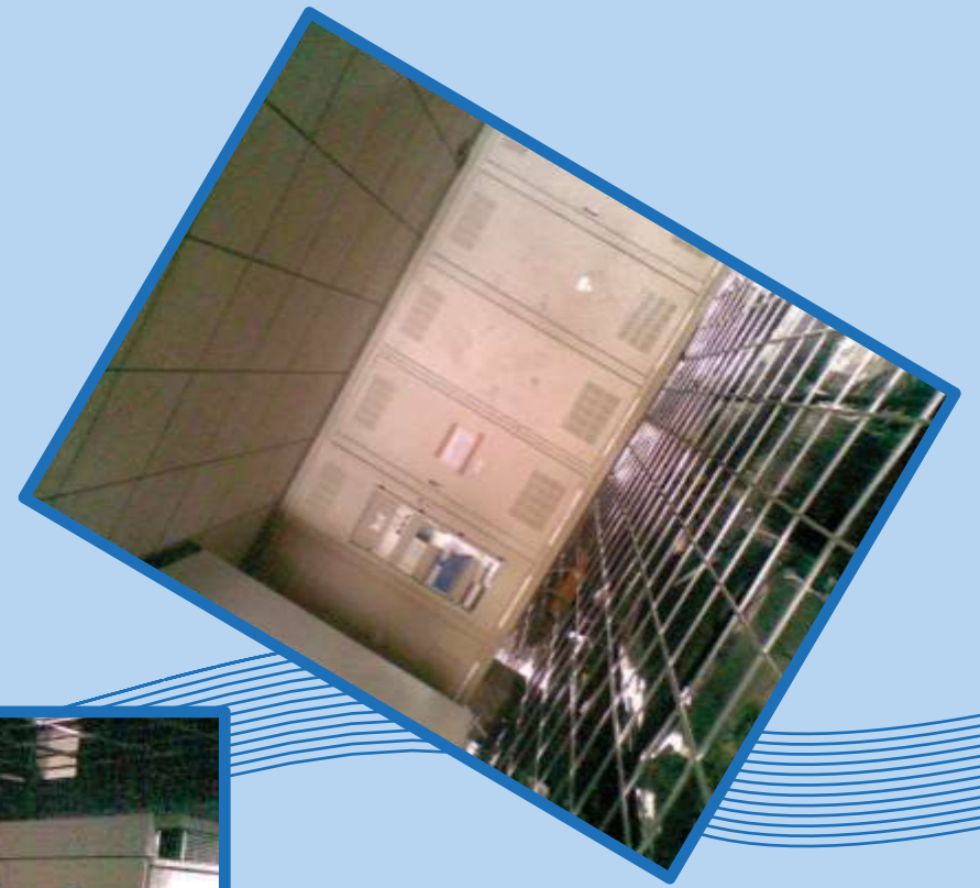
GMR Power Project, Vemagiri, AP
