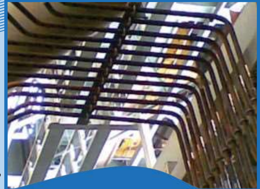
GMR Power Project, Vemagiri, AP
