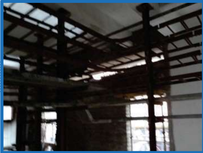
SP- 3& Blast Furnace 8, Bhilai Steel Plant. CG
